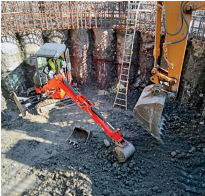
Construction works of a draining well to consolidate the “Fiumicello” ditch slope at km 2+450 of the Sp ex Nsa Bretella di collegamento A3-Ss 585 on behalf of the Province of Potenza
